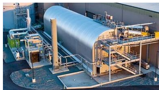
Figure 10-7 Continuous/Plug Flow Digester (Courtesy of Hitachi Zosen Inova)
