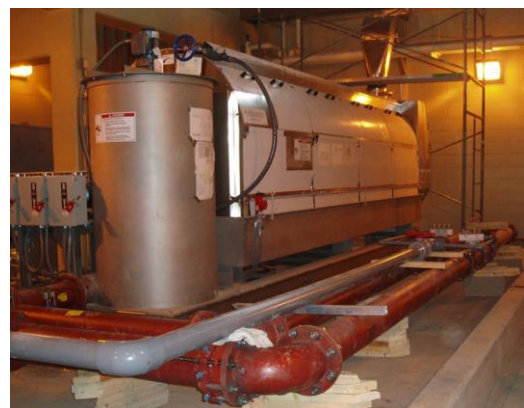
Figure 8-4 Example RDT Installation (Single Drum with Flocculator in Foreground)
