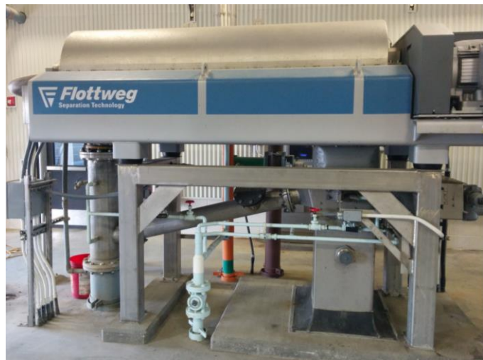
Figure 8-8 Example Centrifuge Installation
