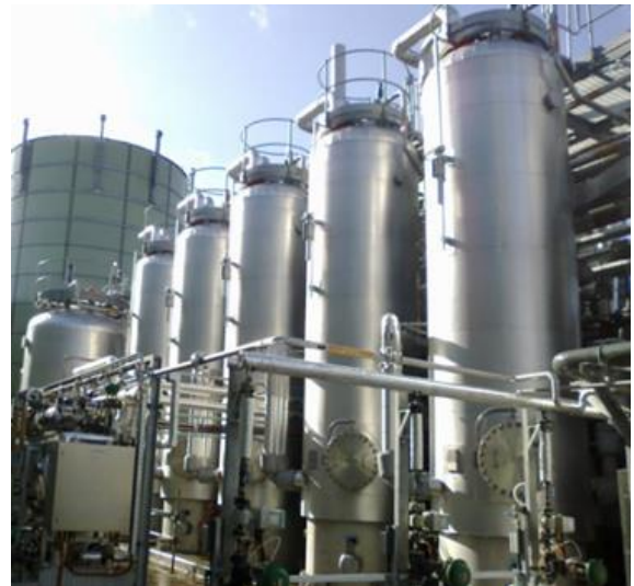
Figure 8-17 Thermal Hydrolysis Process System at Davyhulme, UK
